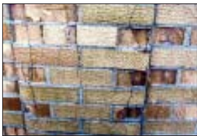
Crumbling brick exterior
